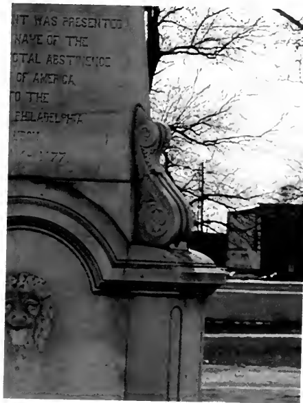
Figure 38: Crack in scrolled bracket (Photograph by author, March 2002)
